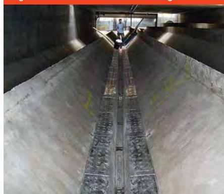
Fig. A.4.5-2 Waste water heat exchanger
