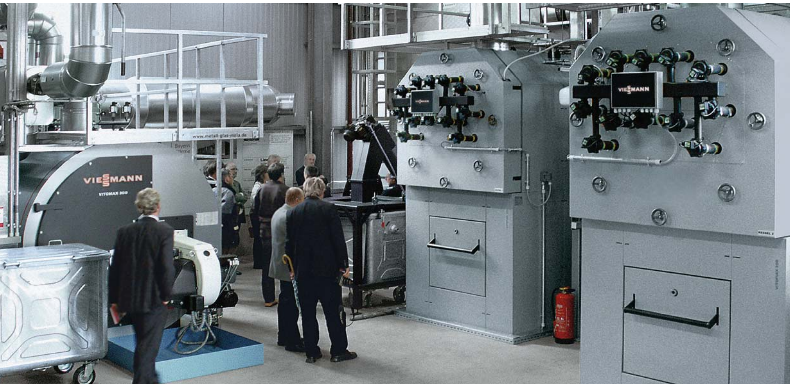
E.ON Biomass Heating Plant Markt Schwaben, Germany
